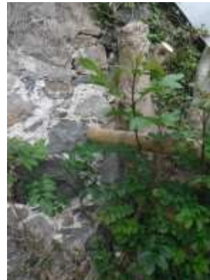
14 - south east elevation - note vertical crack adjacent to tree stump
