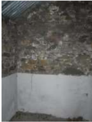
33 - inside of room 1 gable wall - note vertical crack becoming wider with height
