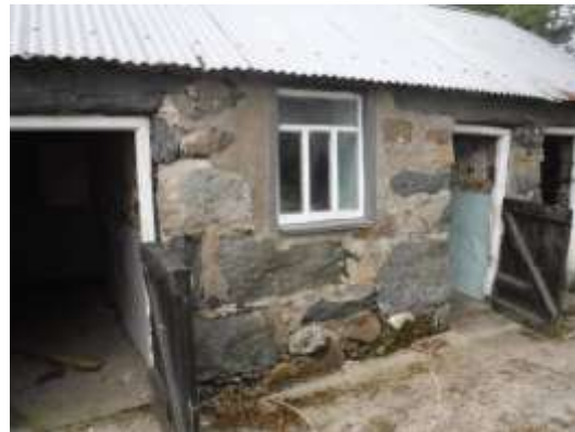
30 - front elevation wall between doors to room 1 and room 2 - note smooth, hard repointing works
