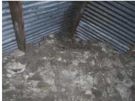
34 - inside of room 1 - external gable pike - note missing stonework
