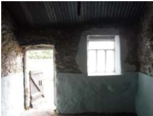
29 - inside of front wall to room 2 - note dropped door frame but square door head
