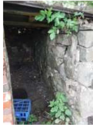
04 - inside of north-west gable wall - note inward bulge local to end of wall
