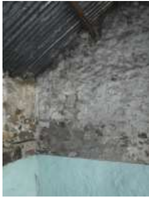
27 - vertical stepped cracking to rear of wall between rooms 2 and 3 - from room 2 - note missing stonework on far side of wall
