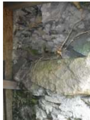
20 - missing stonework to division wall between room 3 and room 2 adjacent to temporary opening
