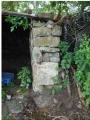
03 - left hand end of north-west gable wall - note slight inward lean
