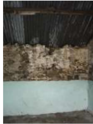
28 - inside of rear wall to room 2 - note uneven eaves level
