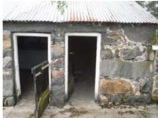
08 - front elevation to Room 02 and room 03 - note slope to left hand door frame does not extend to structural door head which appeared square
