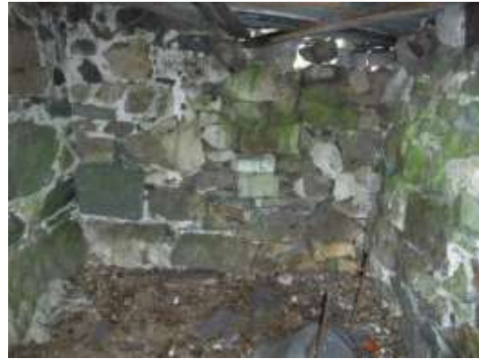
06 - rear wall to room 4 - note loose stone infill to upper right-hand side
